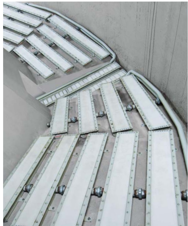
Aeration section and silo outlet
