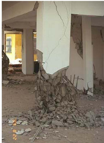
Figure 3-25 Failure of lap splices in a moment frame connection
