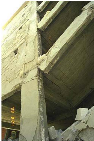
Figure 3-24 Damage to a nonductile reinforced concrete beam
