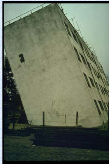
Niigata, Japan earthquake, June 16, 1964 Photo from NISEE
