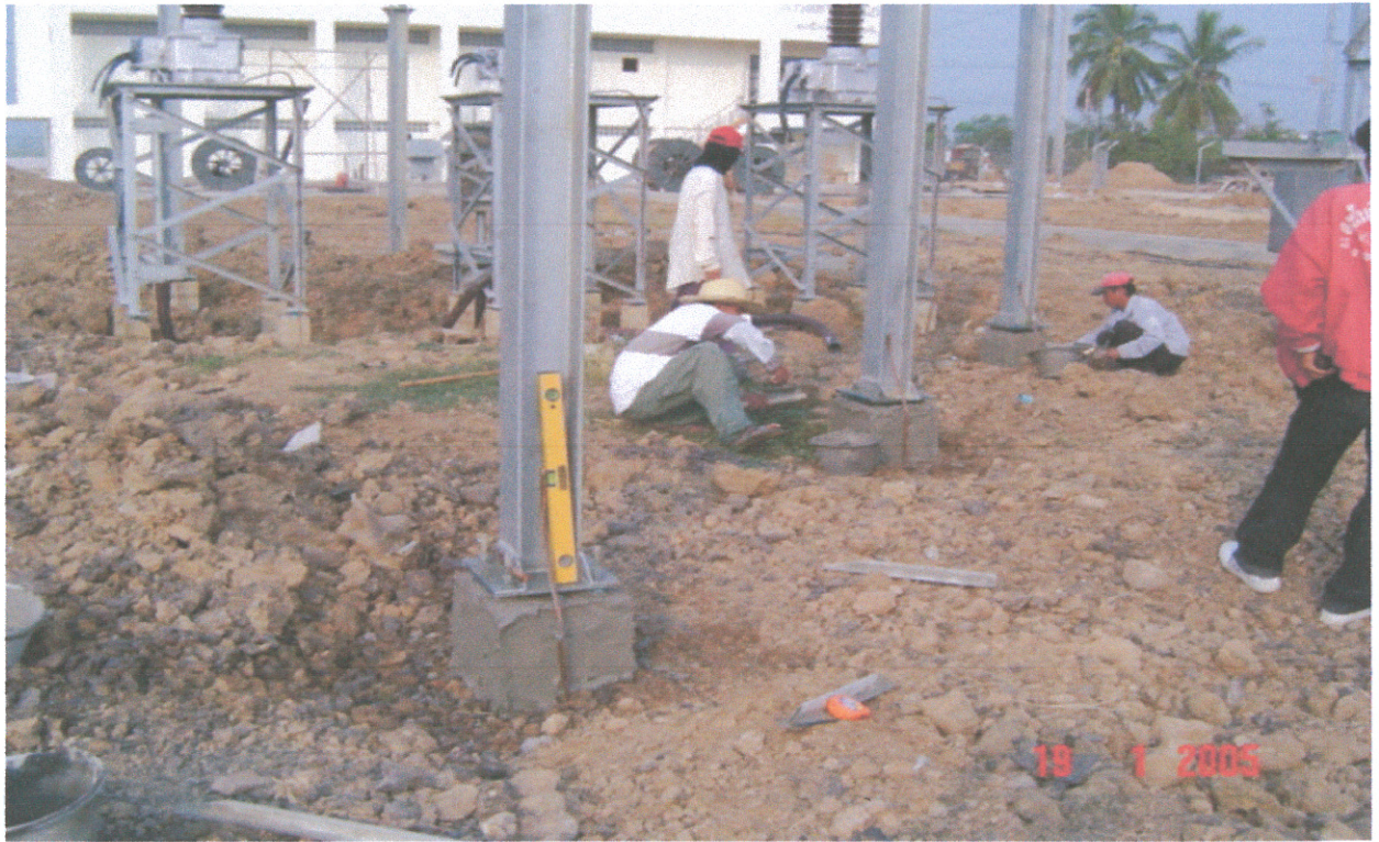
115 KV.BUS POLE SUPPORT
